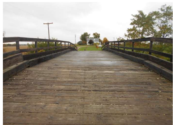
The surface of an old wood bridge near Buda (Robert Tabern photo)
