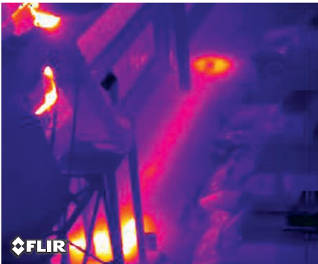
Steam leak underground.
