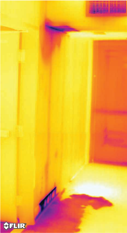
Moisture damage on ceiling, wall, and floor.
