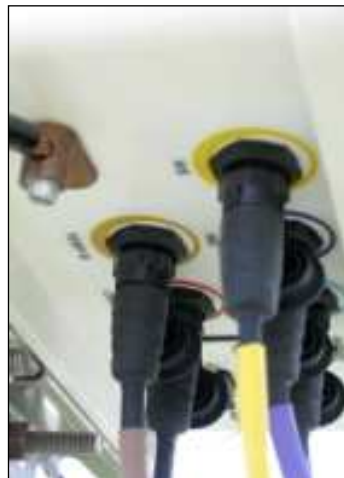
Figure 40: Grounding cable fastened to the ground lug (top left).
