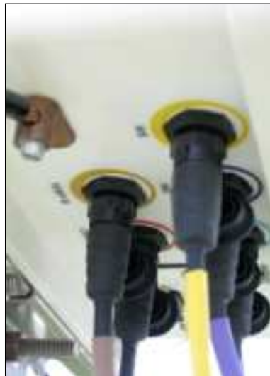
Figure 8: Ground Cable connected to enclosure ground lug (upper left).
