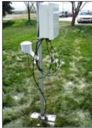
Figure 38: Temperature and RH sensor and enclosure mounted to CM375 Mast.
